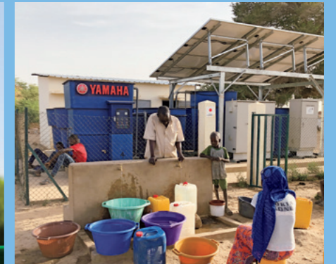
The system is operated independently by a committee formed by the residents.
