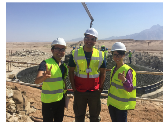
Suganuma (right) managing the progress at the construction site of the wind farm in Egypt, built by Eurus Energy Holdings and others.
